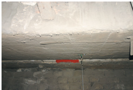
Fig. 4. Registered displacement of ventilation drift relative to the shaft support structure
