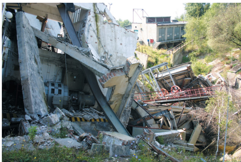
Fig. 1. Construction failure on a shaft object caused by the lack of corrective action
