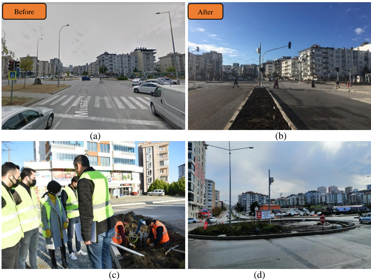
Fig. 2. Real site images for (a-b) before and after transformation and (c-d) construction duration
