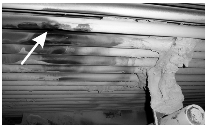
Fig. 1. Superheater failure caused by erosive action of ash carried away with the steam stream of soot blower's jet. Arrow indicates the location of steam leakage
