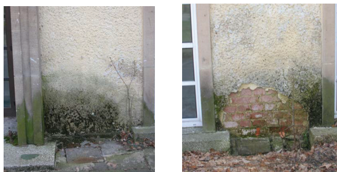
Fig. 1. Walls damaged by dampness
