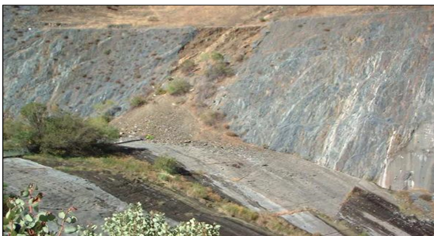
Fig. 9. Real slope failure
