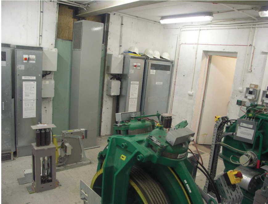
Fig. 3. Machine room with installed gearless winches MX18 with the friction pulleys 690 mm in diameter [3]
