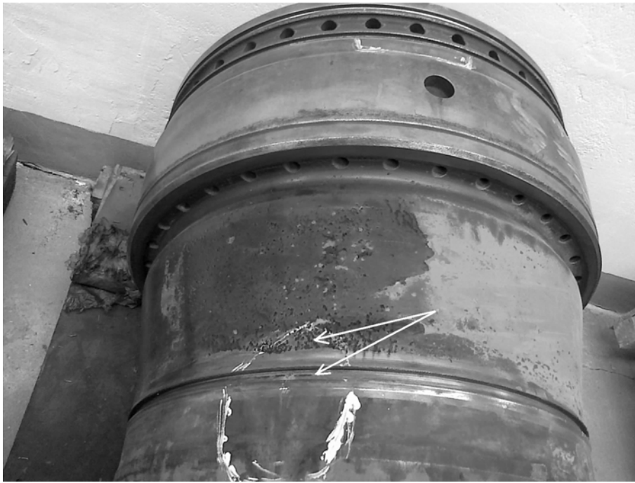
Fig 1. Erosive – corrosive damage to the cooling surface of a cylinder liner of a ship engine of the SULZER 8ZAL 40S type
