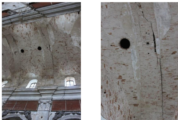
Fig. 5. A view of the cracks and marks on the vault ceiling (photograph to the left), as well as a close-up of the damage (photograph to the right)
