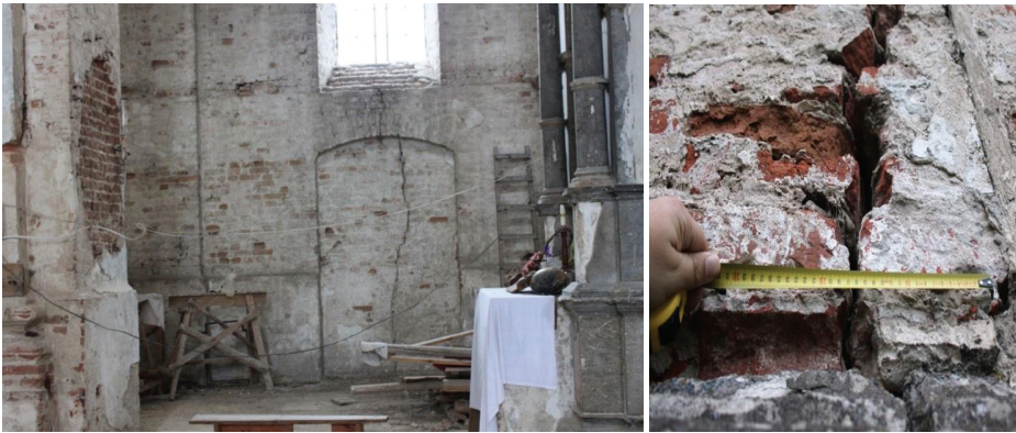
Fig. 6. A view of the damage of the interior wall from inside the building (photograph to the left) as well as a close-up of a visible crack in the structure of the wall (photograph to the right).
