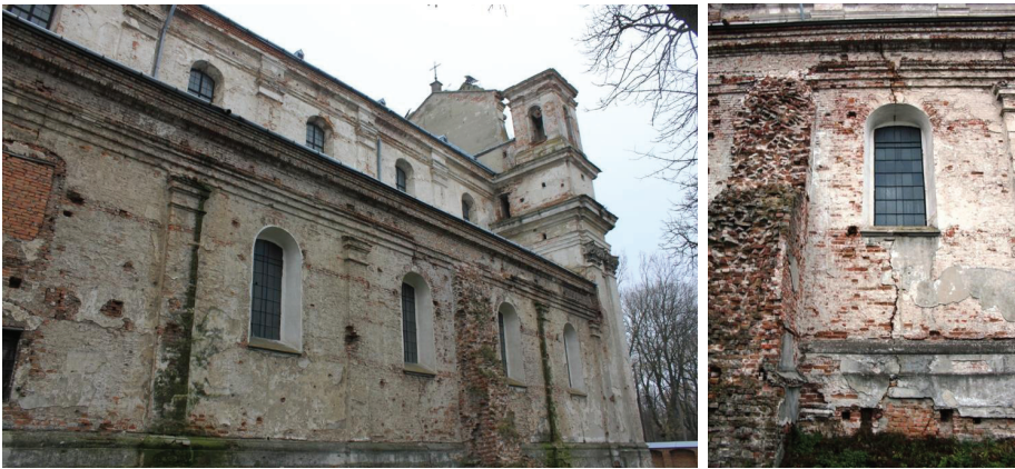
Fig. 7. The photograph depicts the building from the eastern side (photograph to the left). Visible damage of the abutment of the wall, along with the material and structural degradation of the wall (photograph to the right).
