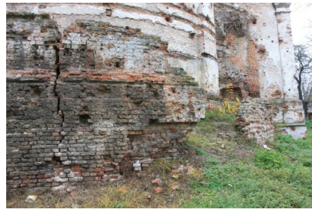
Fig. 11. Losses of mortar within the brick structure of the walls
