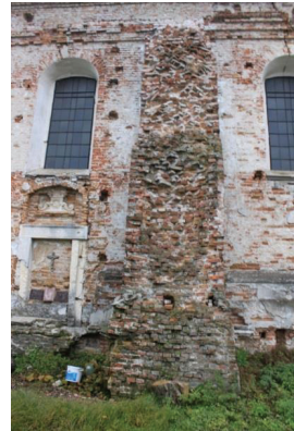
Fig. 9. A damaged abutment. biological corrosion of the walls
