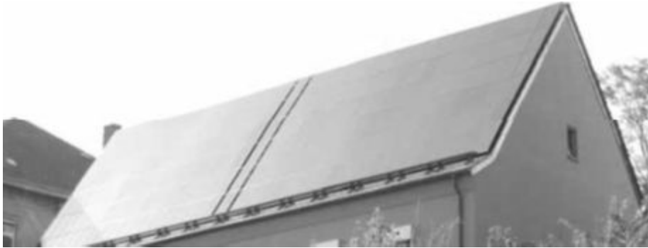
Fig. 10. Roof-mounted CIS installation from the year 2003 on the Fridenskirche church in Tübingen [20]
