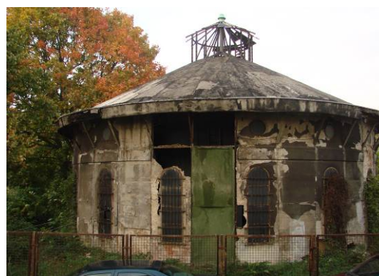
Fig. 3. View of a degraded water tower, 2012 r. Source: author
