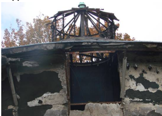
Fig. 6. Steel structure of the wall and roof of a degraded water tower, 2012. Source: author
