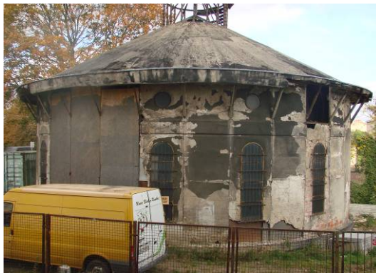
Fig. 9. Fence of a degraded water tower, 2012. Source: author
