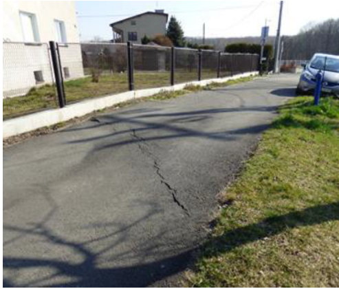
Photo 2. LDGD in the form of steps and fissures 0.05 m wide.
