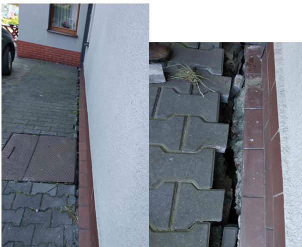
Photo 3. . LDGD in the form of a fissure 0.07 m wide; general view (left), close-up (right).
