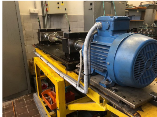
Fig. 2. Three-phase electric motor of Niemann M01
