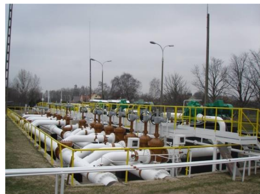
Figure 3. Supporting pumping station in Part A
