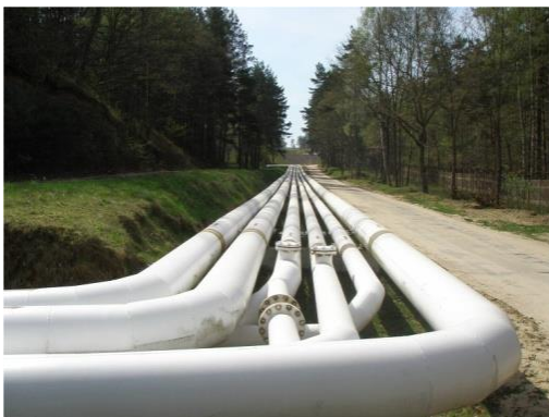
Figure 6. Pipelines in the terminal
