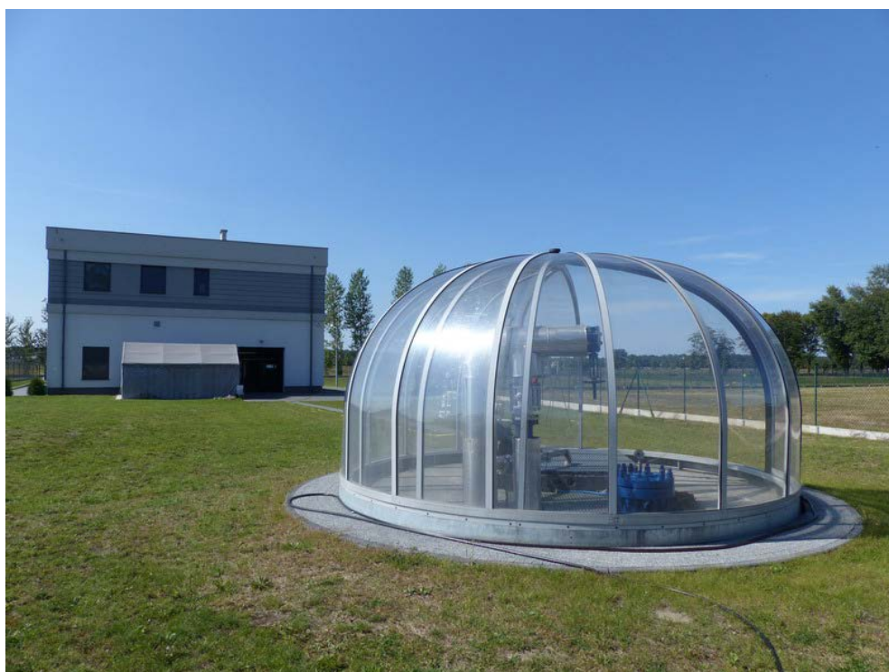
Fig. 3. Geothermal well head (Poddebice GT-2) and heat central in the background
