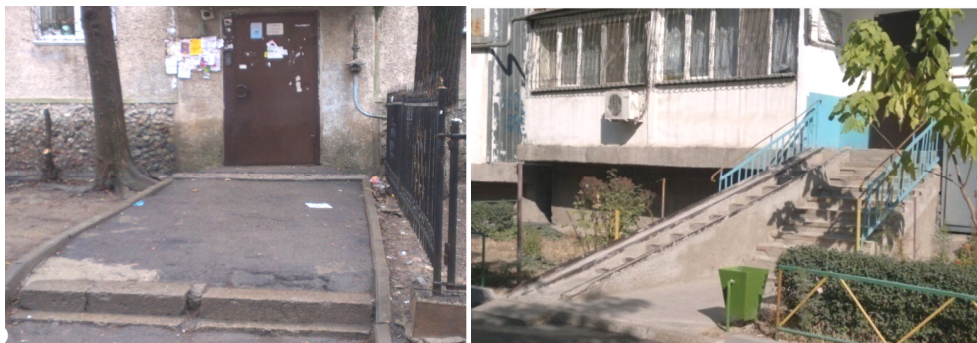
Fig. 3. Analysis of the accessibility of the residential environment on the example of entrance groups of residential apartment buildings in Almaty (Photo: E. Murzagaliyeva)
