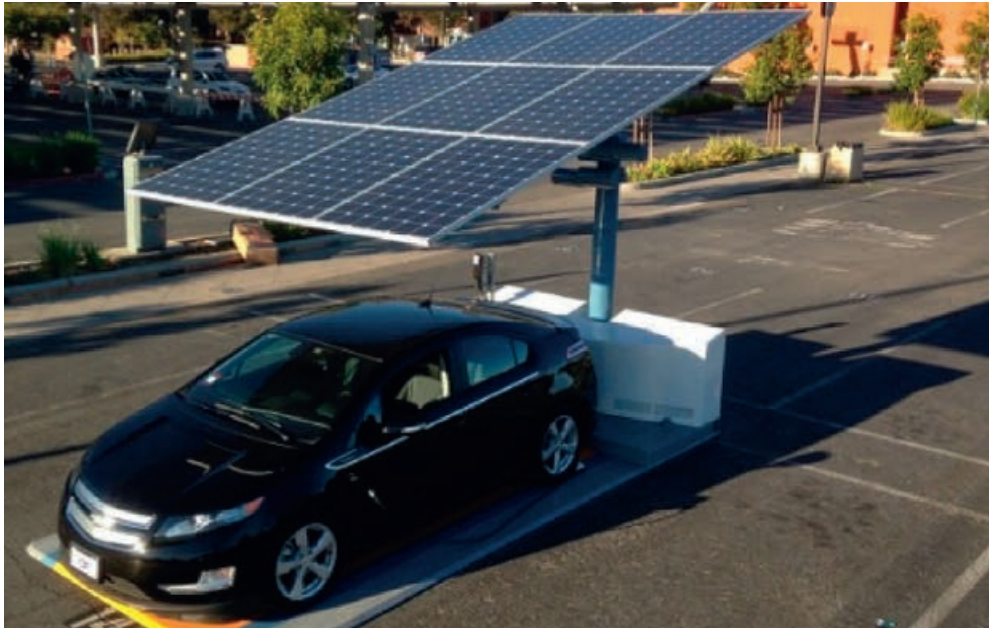
Fig. 1. Autonomous vehicle charging station powered by photovoltaic cells
