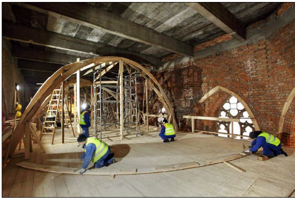
Fig. 7. Installation of centring for the reconstruction of the vault under the existing reinforced concrete ceiling, 2015; photo by L. Okoński.
