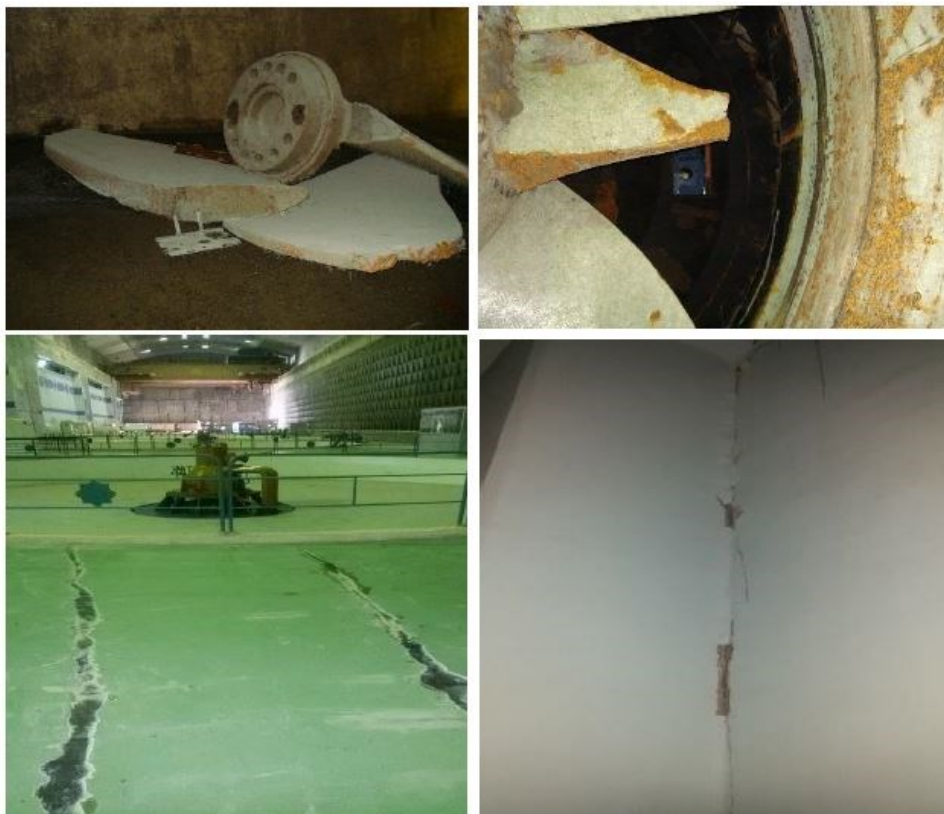
Fig. 1. Runner blade damage (top) and structural cracks in Haditha HPP (bottom)
