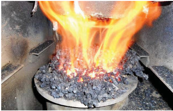
Fig. 3.2. View into the combustion chamber of the heat source during the combustion of alternative pellets
