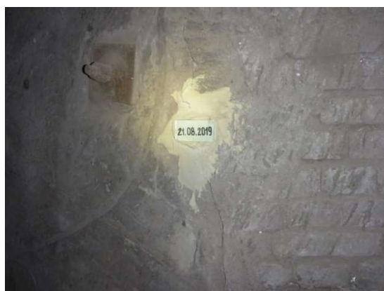
Fig. 1 Vertical crack in the inlet area of the ventilation duct with a applied filling
