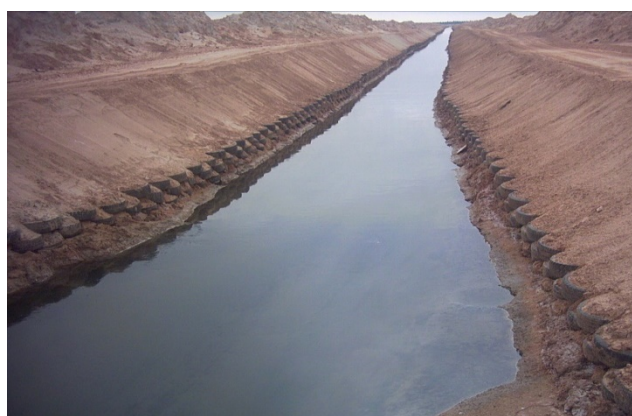
Photo 5. A general view of the magnitude of the channel of Oued Righ (phot. B. Remini)
