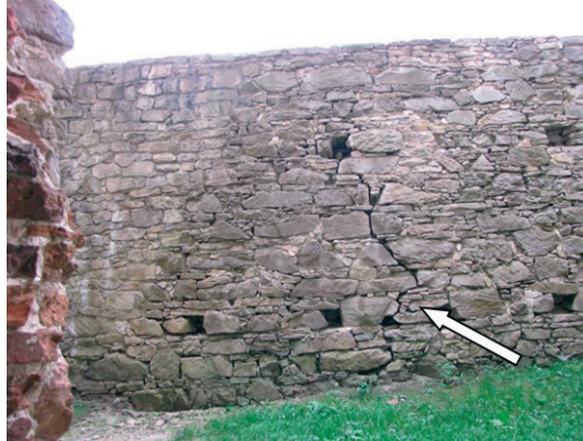
Photo 4. Damage caused by uneven settlement /Krzyżtopór castle in Ujazd/
