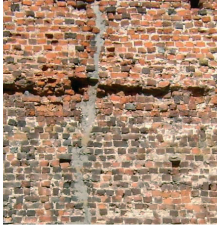
Photo 10. Injection into a crack with a cement mortar (photographer – Sylwester Zieńczuk) /castle in Liwa/
