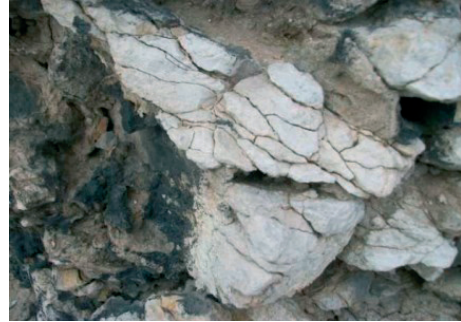
Photo 2. Cracking of a masonry material /castle in Rabsztyń/
