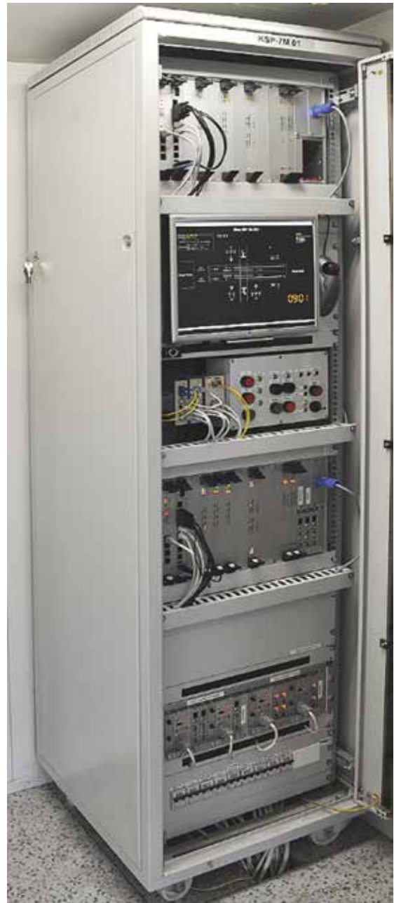
KSP-7M computerized level crossing system
