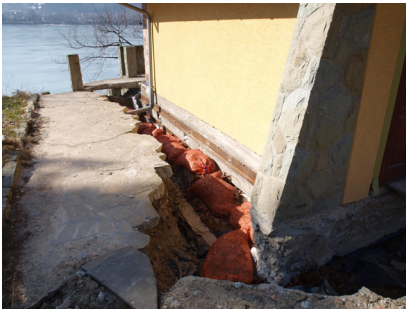
Fig 3. Damage in the houses caused by the movement of the landslide (phot. P. Nescieruk)
