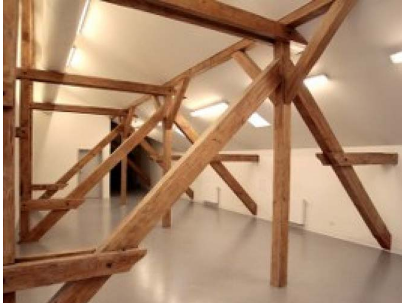
Fig. 18. The exposition of the construction of a timber roof truss in the attic, the front bay of the building, 2015. Source: photog. by M. Tuszyński
