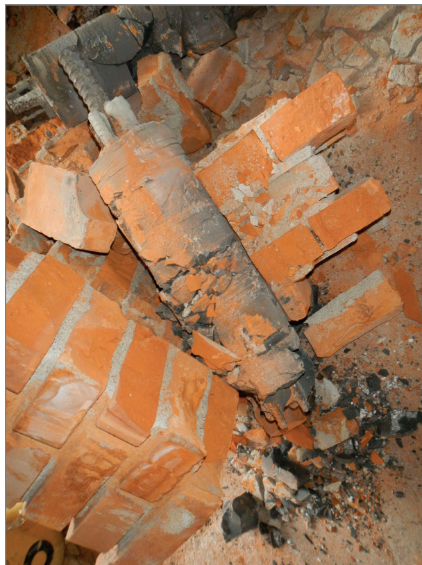
Photo 14. Damaged masonry foundation specimen
