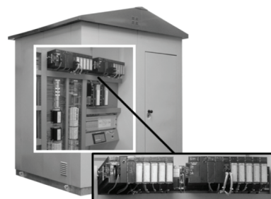
Fig. 1. The view of two channel structure of cross level protection system, type RASP-4
