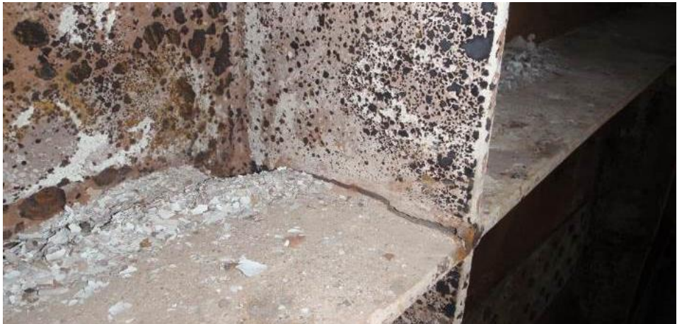
Fig. 9. Typical crack of weld
