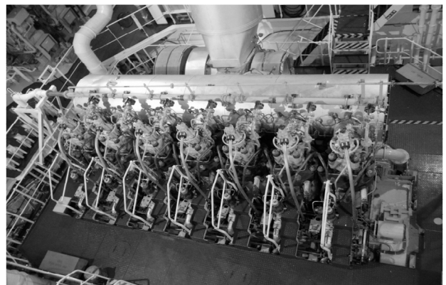
Fig. 1. Engine MAN B&W 7S50MC-C from upper platform of engine room
