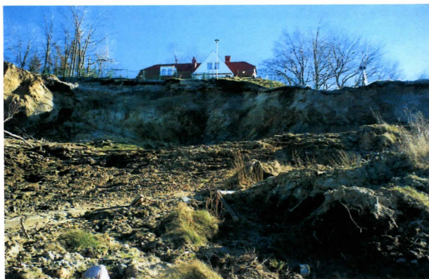
Fig. 2. Landslide viewed from the level of coluvium – spring 1999
