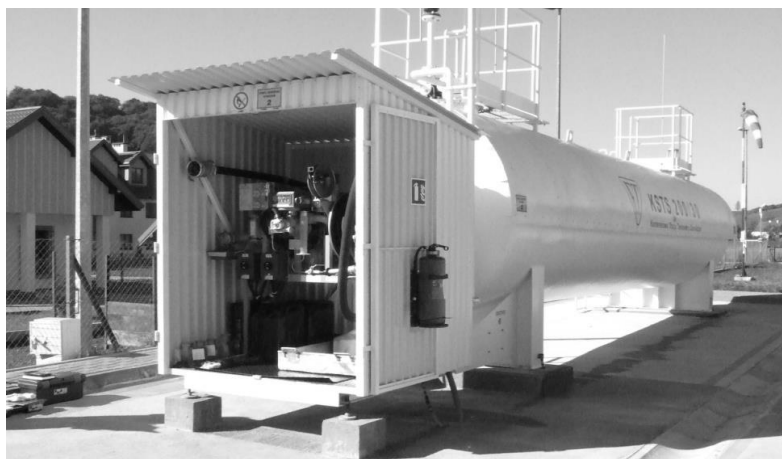
Fig. 4. Border Guard landing area - an aircraft refuelling station with a capacity of 30,000 l, equipped with a distribution node
