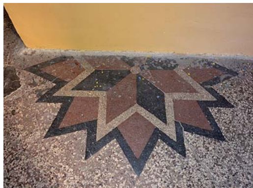
Fig. 31. The terrazzo floor with star ornament divided with later constructed wall. Source: photo by author
