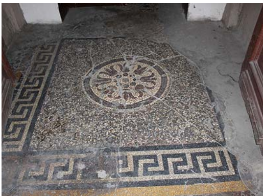
Fig. 30. The destruction of terrazzo floor in the vestibule in 20 Lepkoho Str. Source: photo by author
