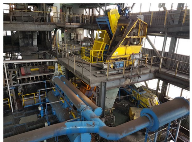
Fig. 5 ZG "Sobieski" bucket conveyors Source: [33].
