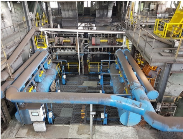
Fig. 1 Two pulsatory jigs OM15, ZG "Sobieski" Source: [33].
