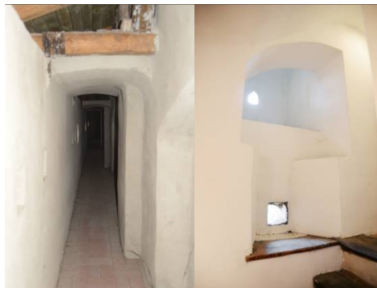
Fig. 6. The corridor with battlements over the arcades (on the left) and battlements in the church tower (on the right, the Author's photography)
