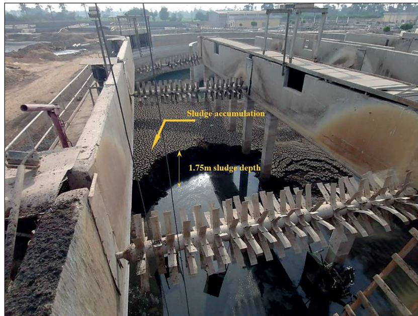
Figure 1. Sludge accumulation inside the oxidation ditches
