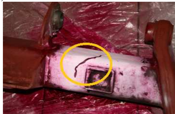
Fig. 6. View of BPW axle of semi-trailer with suspicion of cracks (a) and detected crack by penetrant method (b) [7]
