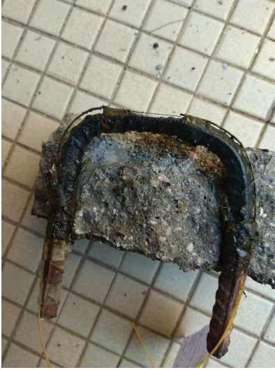
Fig. 4. The rusts on the steel bars.
