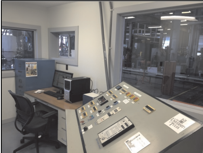
Fig. 3. TUDRP Rig. Control Room: PC-based data logger and control panel
