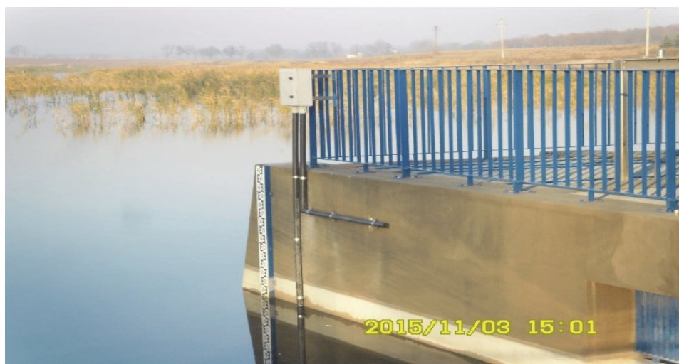
Fig. 2. A staff gauge with a hydrostatic probe installed at the damming structure at the outflow from the reservoir
