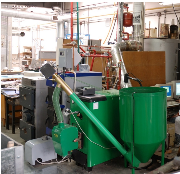
Fig. 3. View of the heat station located in a laboratory belonging to the Poznan University of Technology (Division of Heating, Air Conditioning and Air Protection, Institute of Environmental Engineering)
