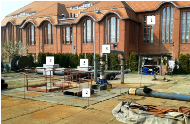
Fig. 2. The area of Gliwice II shaft. 1 – the building of Higher School of Economy in Gliwice, 2 – two symmetrical points of emission, 3 – pipelines for water pumps, 4 – the outlet of the fan no. 1, 5 – the outlet of the fan no. 2
