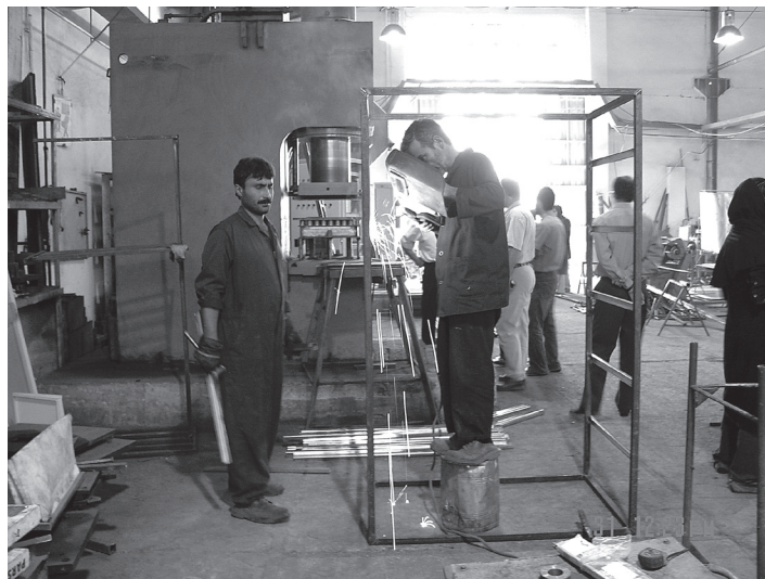
Figure 5. Worksite before improvement: no personal protective equipment for welder and coworkers, poor posture.
