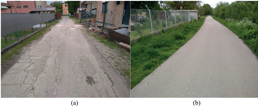
Fig. 6. The residential streets with different road surface quality: (a) cracked asphalt, (b) smooth asphalt
