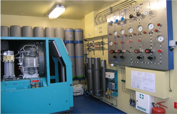
Fig. 20 General view of the interior of the Mobile Air Supply Set. Source: own study.
