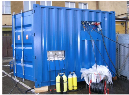
Fig. 23 General view of the supply system for an ORTOLAN base securing underwater works. Source: own study.
