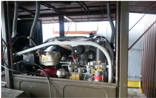
Fig. 22 View of the interior of the supply system for an ORTOLAN base securing underwater works equipped in MARINER 320 D compressors. Source: own study.
