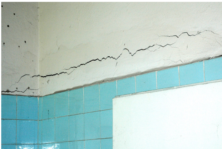
Fig. 10. Horizontal cracks in masonry partitions in basements. Source: author
