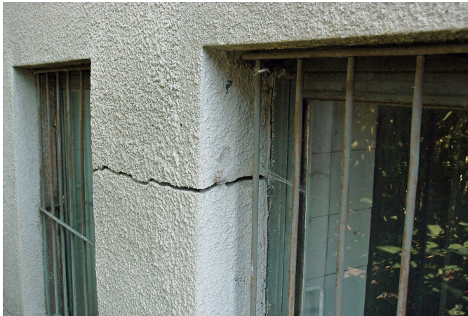
Fig. 9. Fragment of the basement wall of segment 1 – visible cracks in the inter-window pillar from the outside and no damage at this point inside. Source: author
