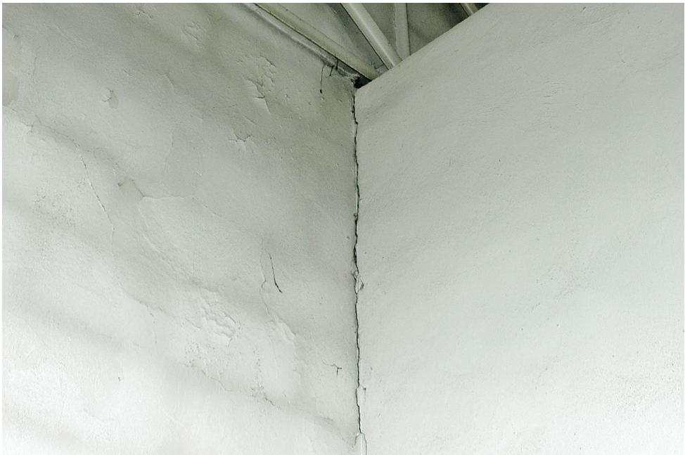
Fig. 11. Cracks at the junction of the masonry partition wall of the second storey with the western gable wall. Source: author
