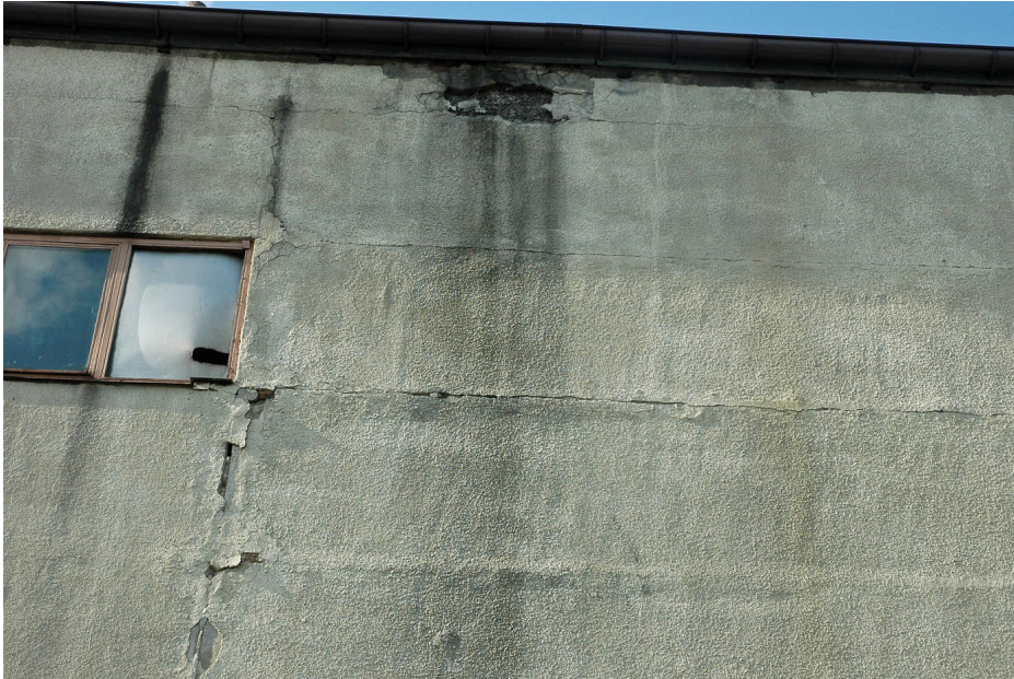
Fig. 12. Western fragment of the northern wall of segment 1 – visible cracks and chipping cracks and chipping of plaster at the joints of prefabricated housing elements and dark damp patches. Source: author
