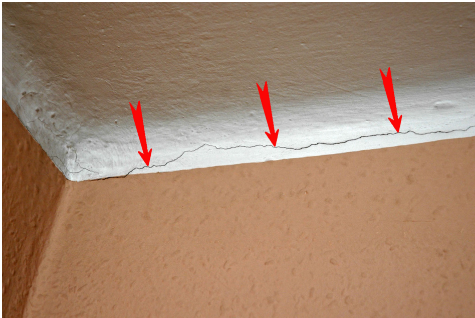
Fig. 6. Gap of up to 1.5 mm between ceiling and first floor interior wall. Source: author
