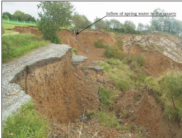
Fig. 3. Region of the landslide main scarp. An inflow of water from a spring into the landslide area can be seen
