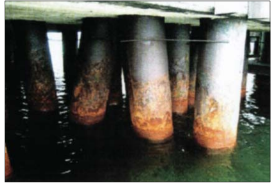
Fig. 6. Sea corrosion of piles [10]
