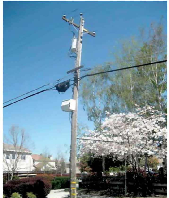
Fig. 2. Low voltage distribution network in the residential district of Danville, near San Francisco
