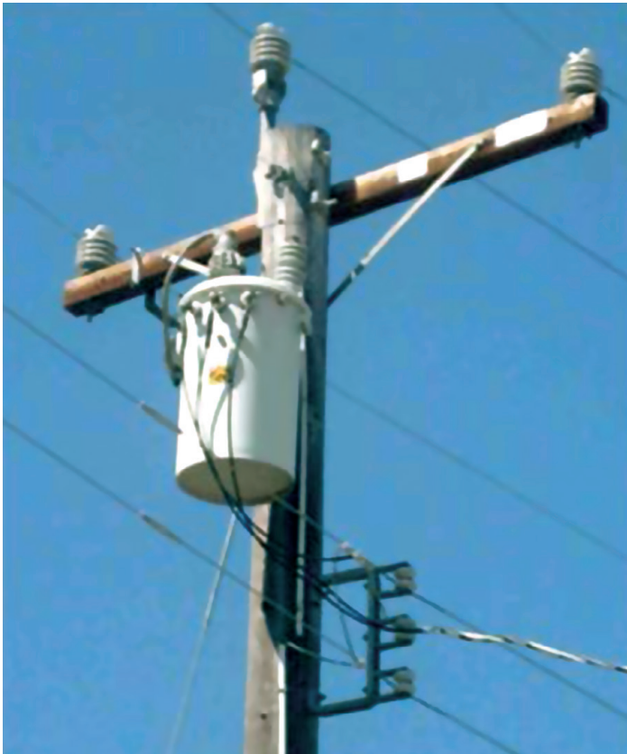
Fig. 1. High voltage distribution grid in the residential district of Danville, near San Francisco
