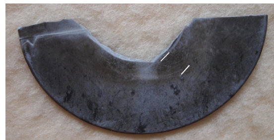
Fig. 9. The upper surface of the Lt insulator middle shed sample. The lines denote the area under examination with a bigger intensity of and small cracks in the dark coating. The measurement was taken towards the shed edge
