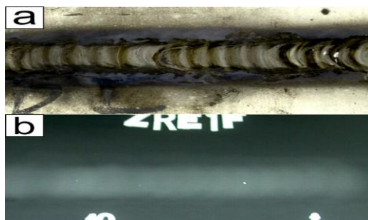
Fig. 5. Results of visual inspections of welded joint marked as Z2: a) face of welded joint (3,0 kJ/cm) b) radiograph of welded joint
